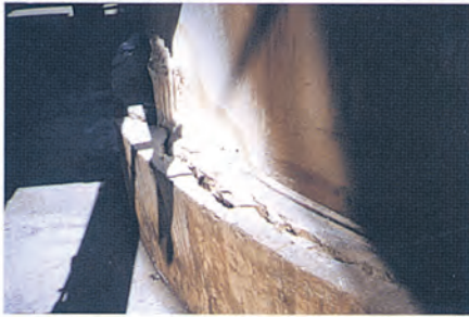
Cracked and spalled tank base
