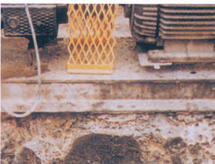
A deteriorated pump base
