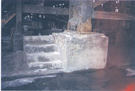
Deteriorated pedestal for main support beam
