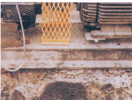
A deteriorated pump base
