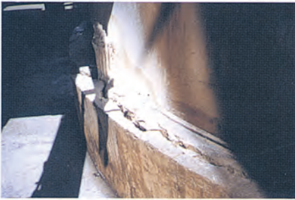
Cracked and spalled tank base
