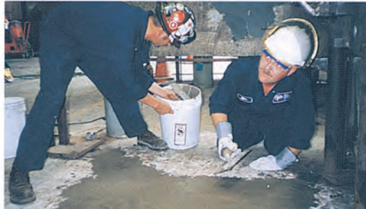
Badly spalled floor area being prepared with a high strength repair material.
