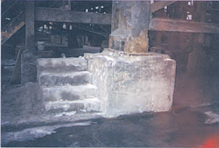
Deteriorated pedestal for main support beam
