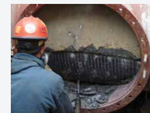
Steel cylinder and concrete wires exposed
