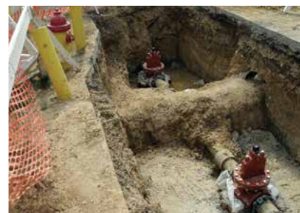
InsertValves on AC pipe for main control and hydrant replacement preventing asbestos fibers becoming airborne
