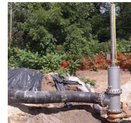
36" force main line stop with internal 24" bypass
