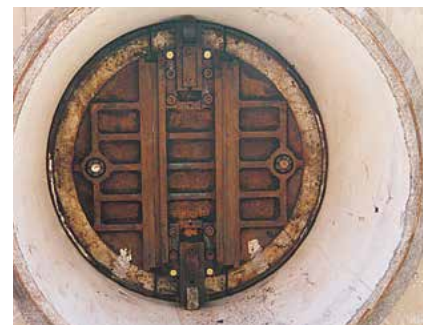
FOLDING HEAD SYSTEM Sequence of 36" (ND 900mm) folding head installed in steel cylinder reinforced concrete test pipe
