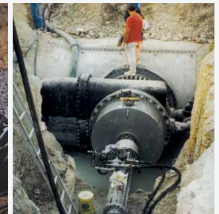
60" Tap on SP-12 concrete pipe
