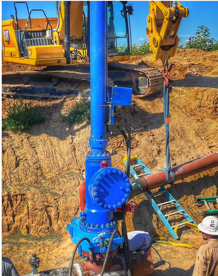
Figure 3. SmartStop providing isolation for a new tie-in.
